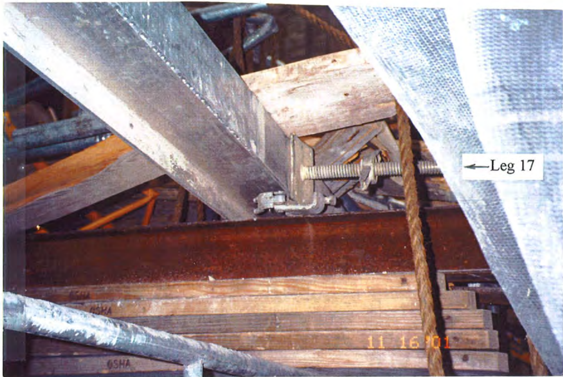
Figure 3-25. The Rotational Failure of Leg 17 above the South Top Horizontal Member of the Offset Scaffold (Looking Toward East).
