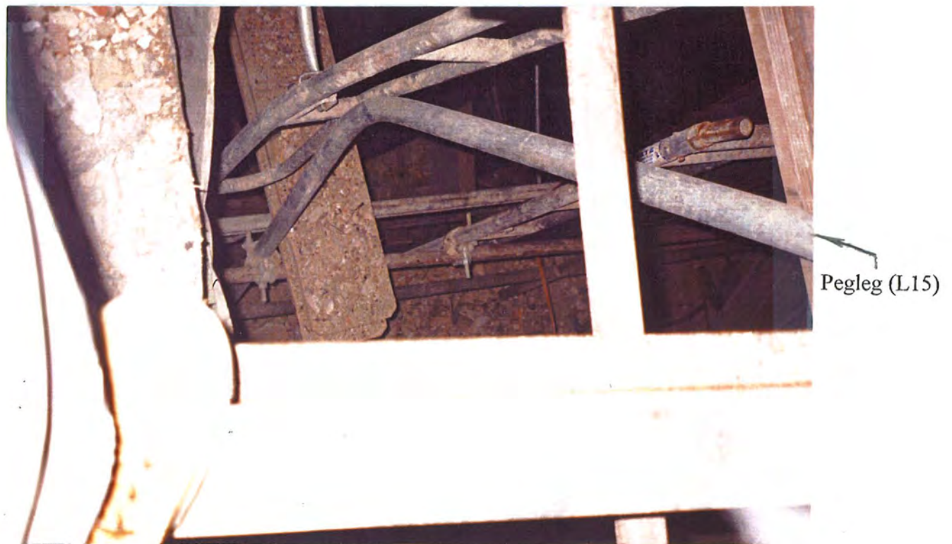
Figure 3-20. Failed Condition of the Pegleg with no Bent at the Lower Connection to the Handrail (Looking Downward from Top).
