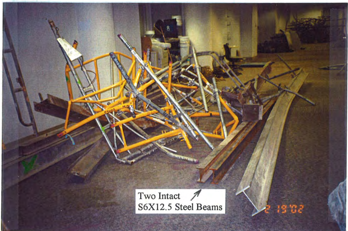
Figure 3-28. Condition of the Recovered Scaffold Frames, Lateral Bracings, and Bottom Support Members II.
