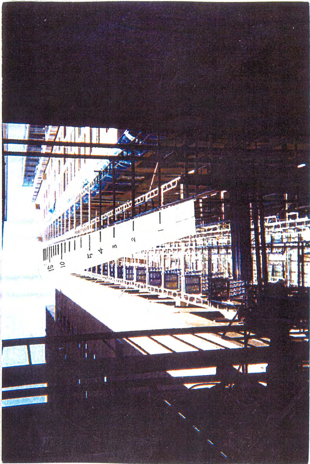
Figure A-2. Two Scaffold Planks Stuck out on the South End of the East Tower at the 19 th Level (from Scaffold Erector).
