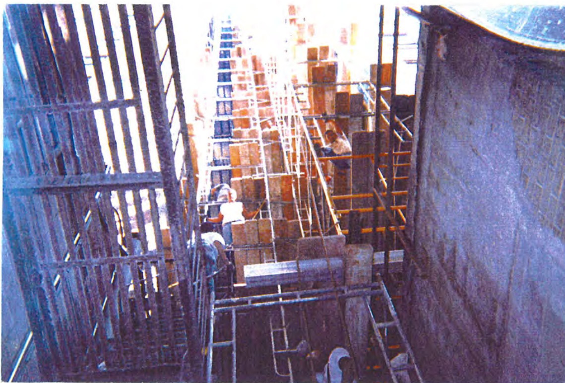
Figure 3-10. Support Conditions at the Base of the Southern Portion of the Scaffold Towers II (from Scaffold Erector, Looking Toward North and Upward).
