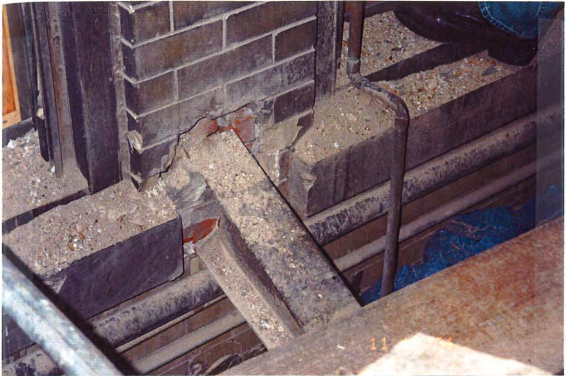
Figure 3-15. Collapsed Condition of Dunnage No. 2 at West End.
