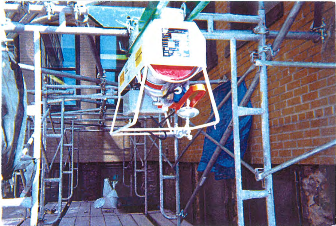
Figure 3-12. Lateral Bracing Conditions at the Top of the Scaffold Towers II (from Scaffold Erector, Looking Toward North). Note that the electrical hoist in the upper middle of this figure was mounted on top of the southmost bay of the east tower prior to the collapse.
