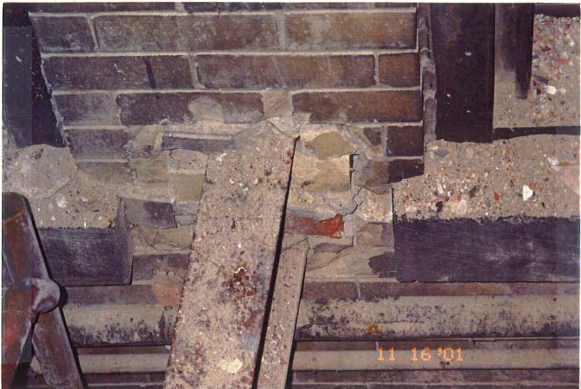
Figure 3-17. Collapsed Condition of Dunnage No. 3 at West End.
