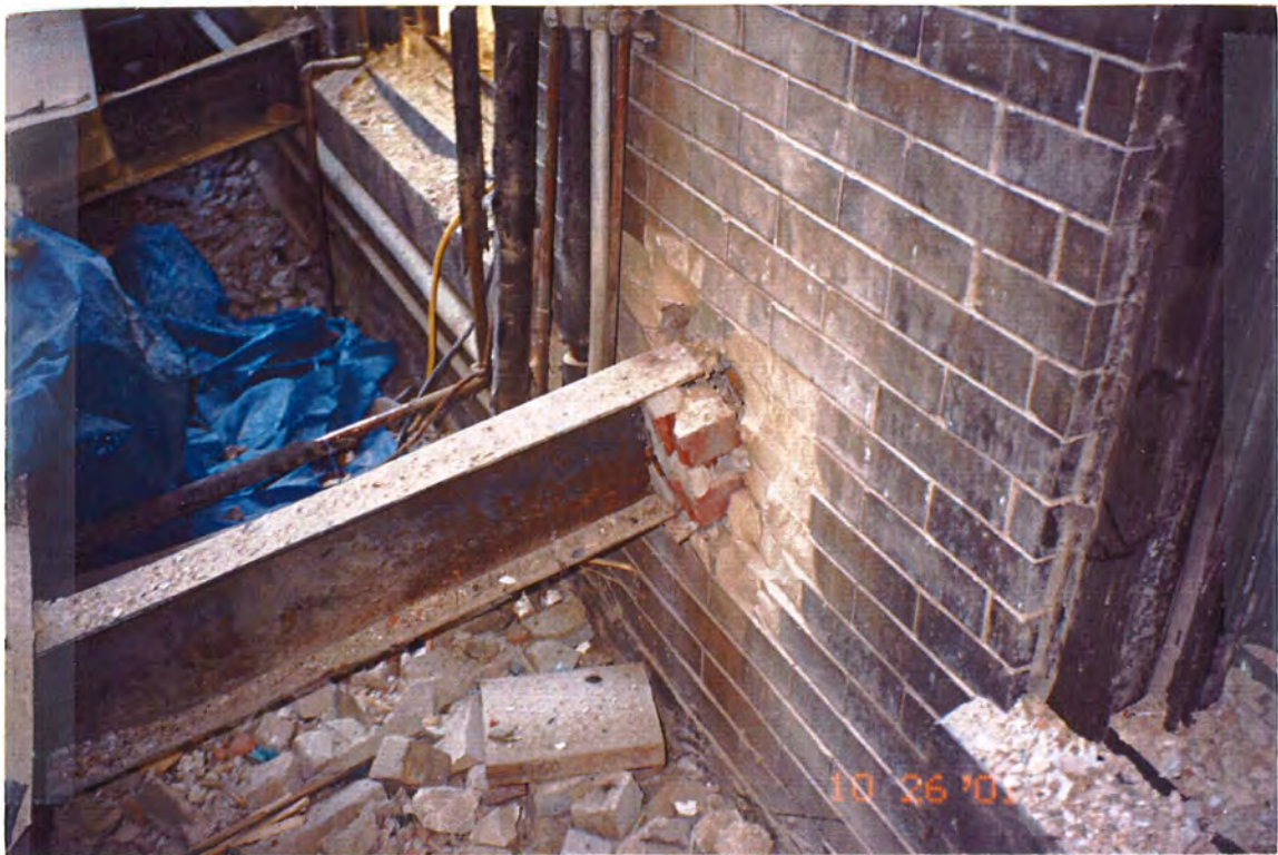
Figure 3-13. Collapsed Condition of Dunnage No. 1 at West End.
