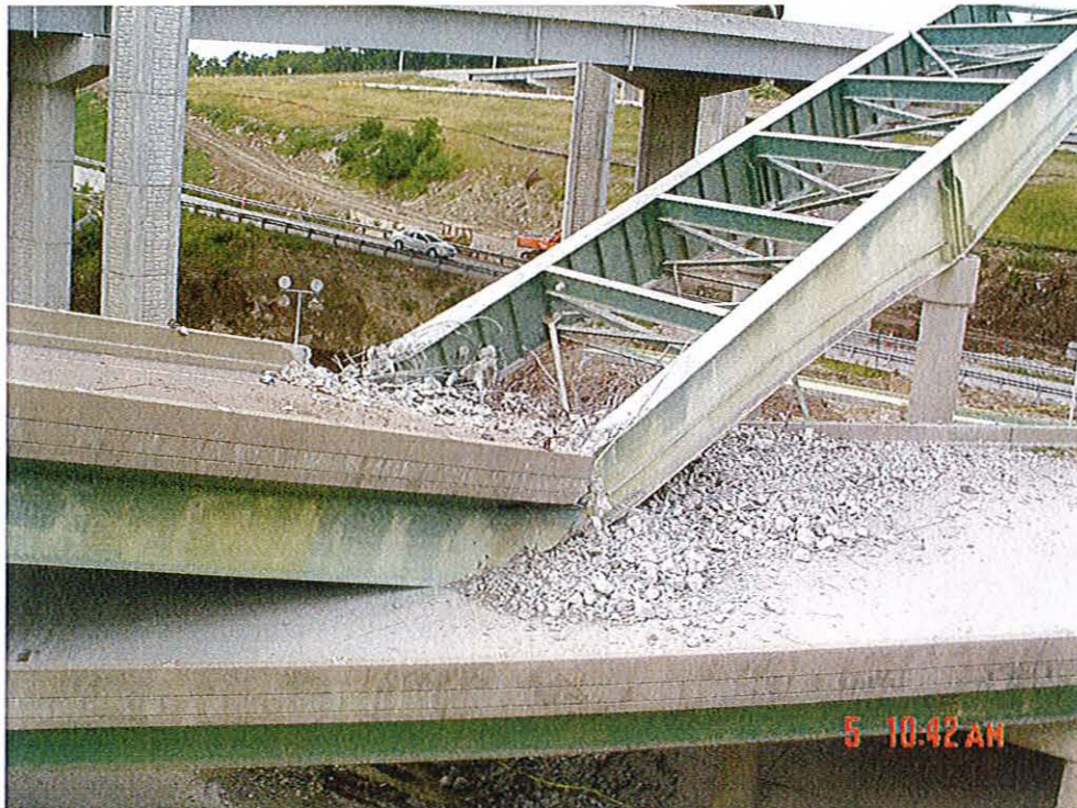
FIGURE 14 (Looking south, collapsed bridge girder span 2-3 fell on lower bridge into V-shape)
