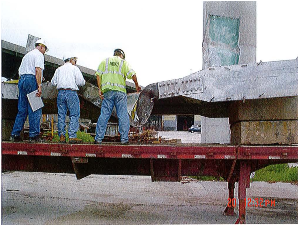
FIGURE 24 (Twisted top flange of the girder)
