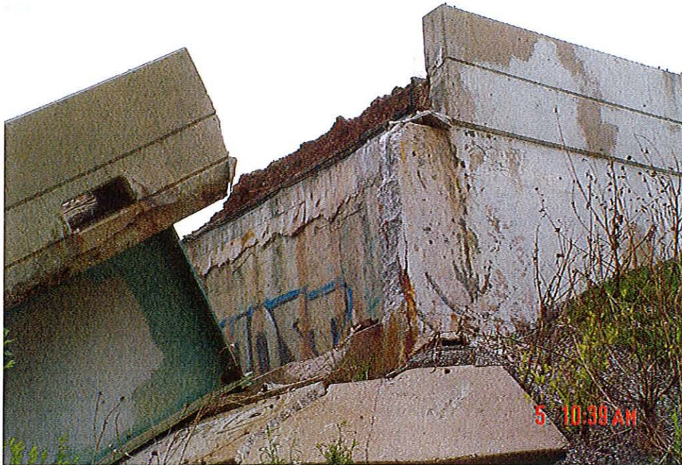
FIGURE 11 (Looking north, bridge girder separated from bent no. 1 abutment)
