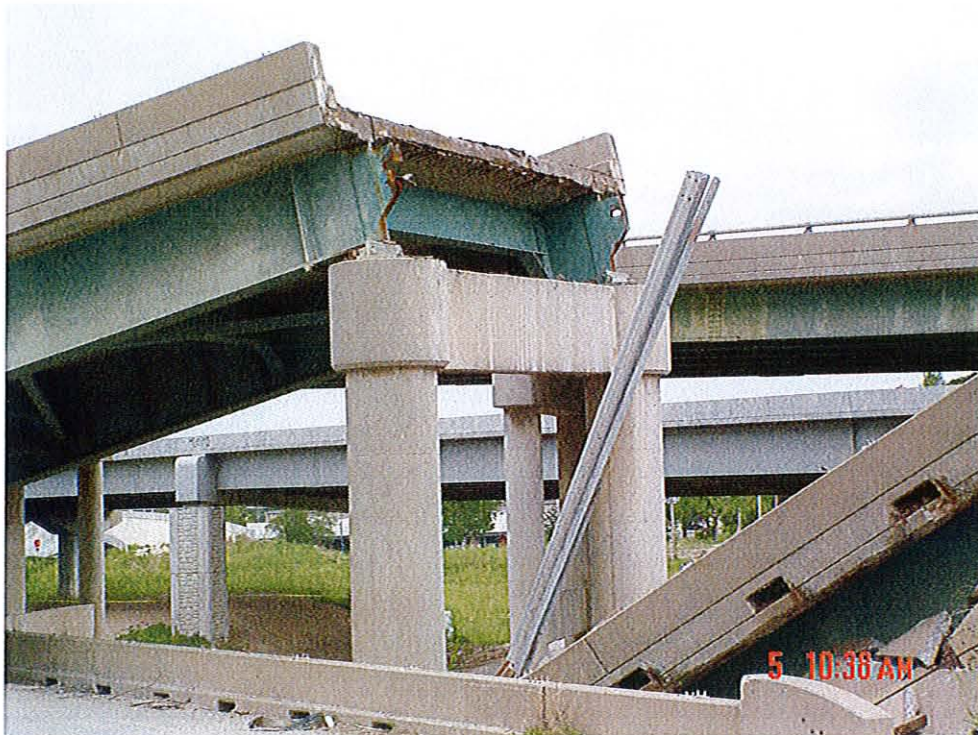
FIGURE 12 (Looking north, bridge girder at span 1 separated from pinned connection near bent no. 2)
