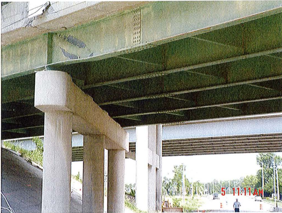
FIGURE 19 (damage to lower bridge girder framing due to upper bridge collapse)
