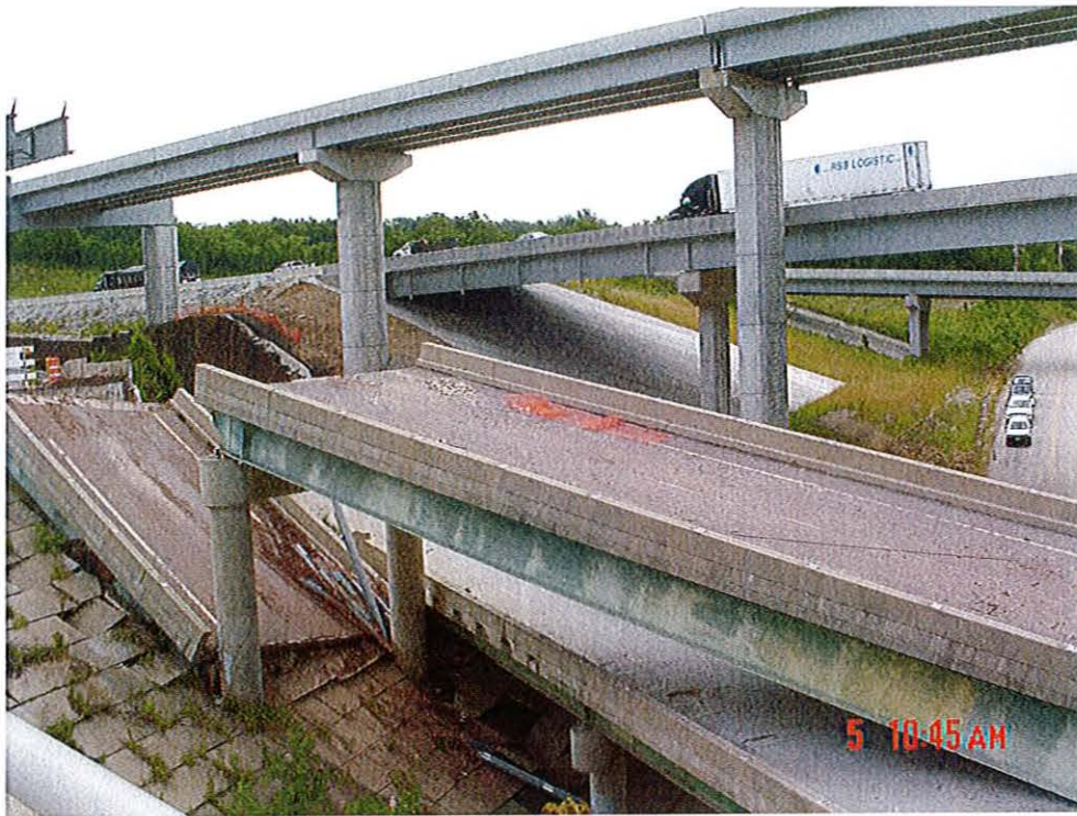
FIGURE 15 (Looking south, Separation of bridge girder near bent no. 2)
