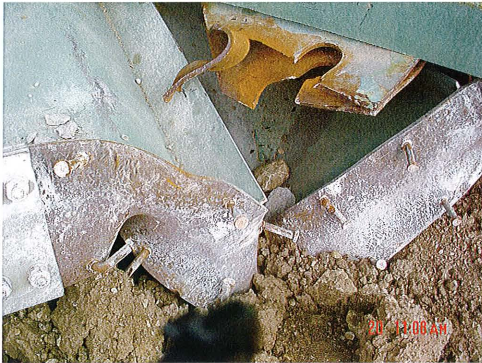
FIGURE 22 (Damaged top flange of the bridge girder)
