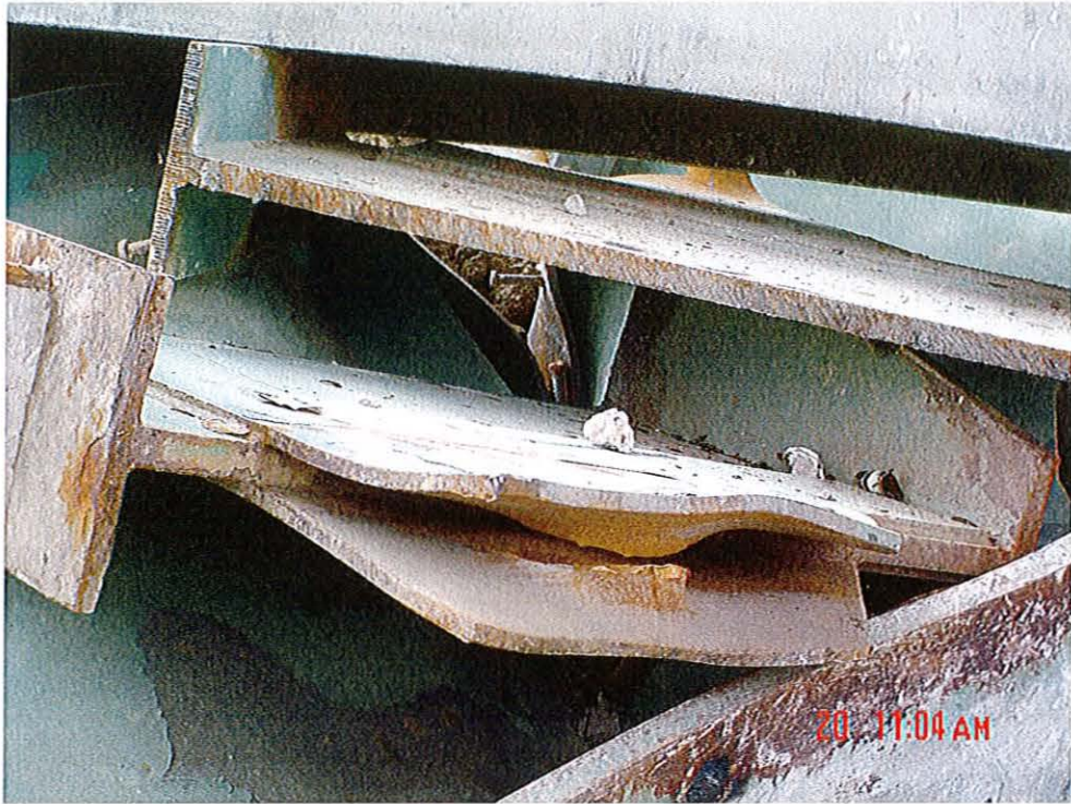
FIGURE 21 (Damaged top flange of the bridge girder)
