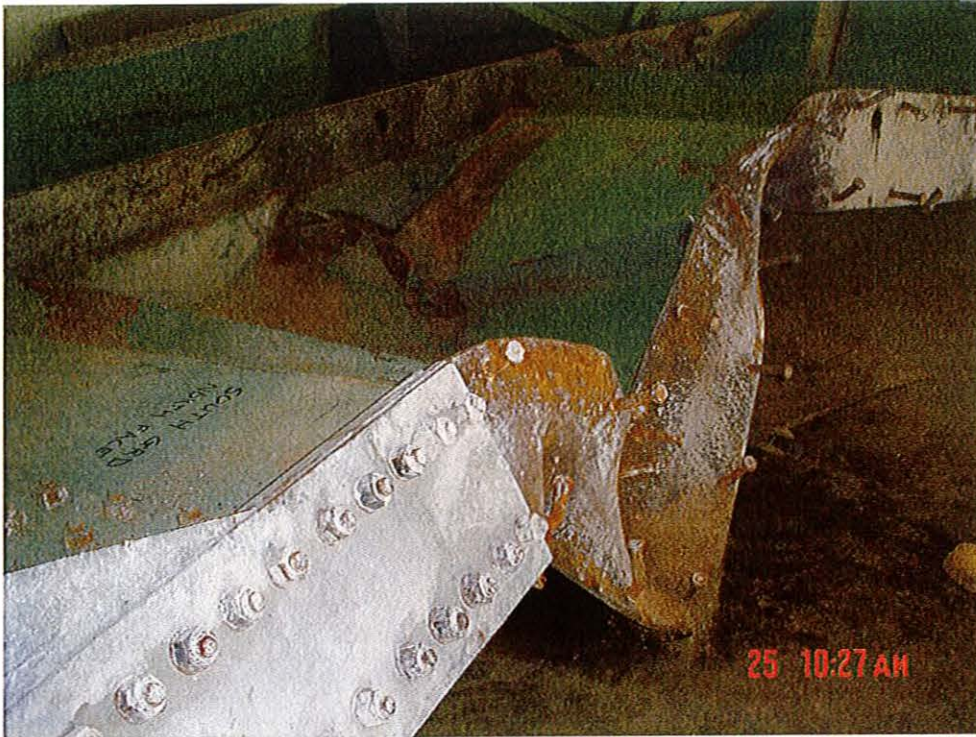
FIGURE 26 (Twisted top flange of the south girder)
