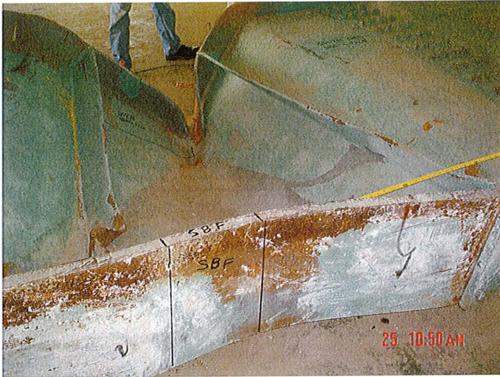
FIGURE 32 (South girder bottom flange)
