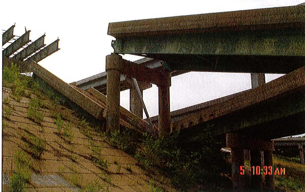
FIGURE 5 (Looking south, collapsed bridge girder between bent no. 1 & 2)
