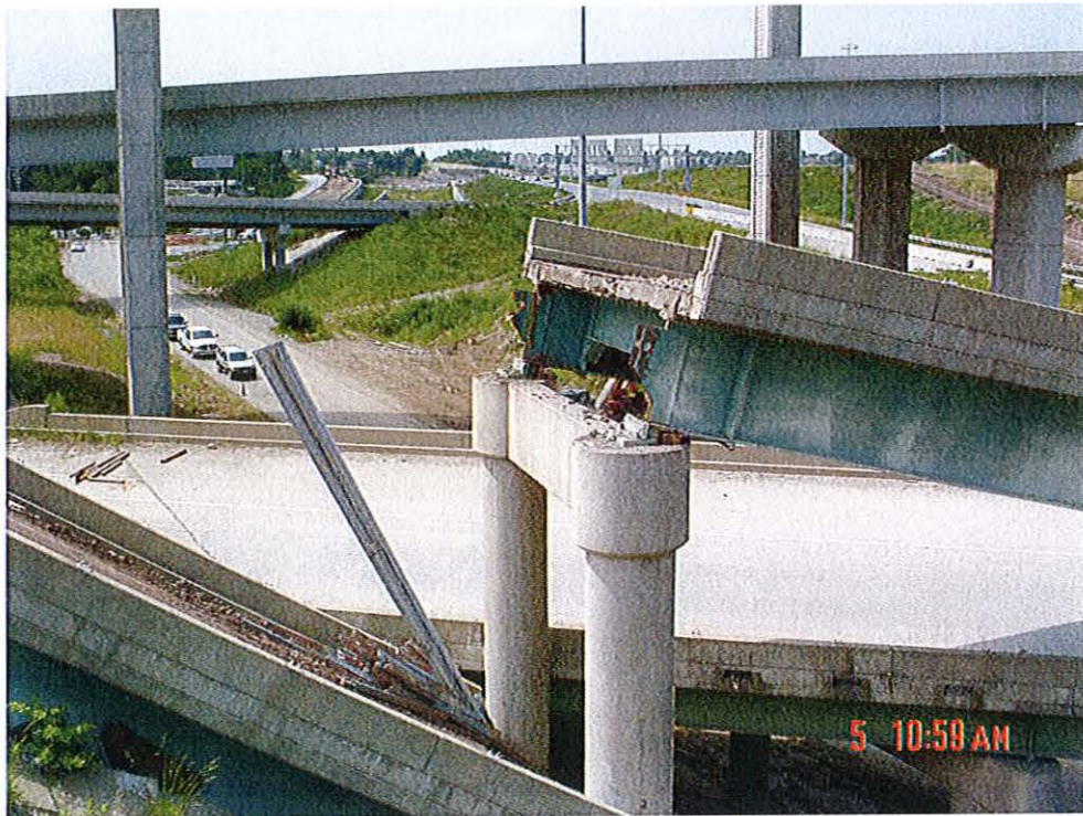
FIGURE 18 (Looking south, Separation of bridge girder near bent no. 2)
