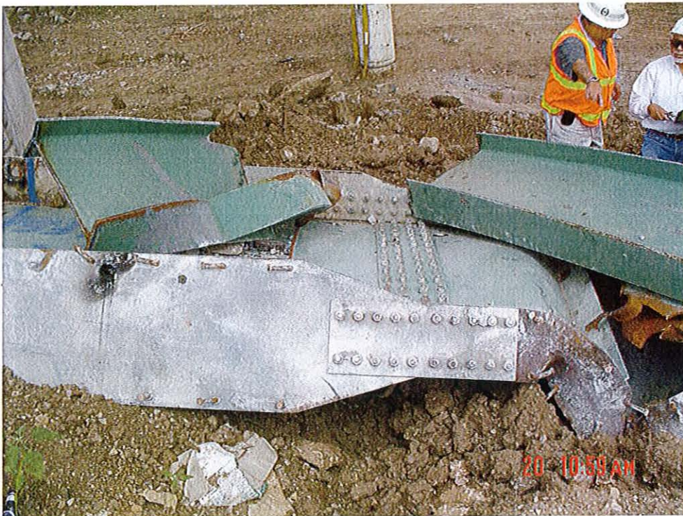
FIGURE 20 (Damaged top flange of the bridge girder)
