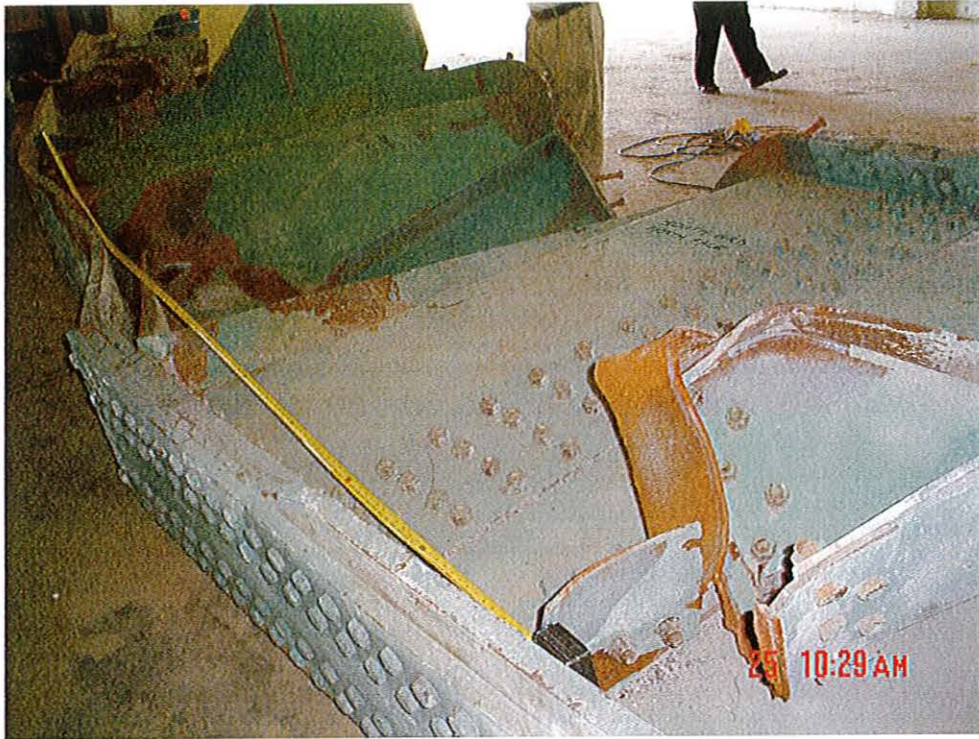
FIGURE 28 (South girder bottom flange)
