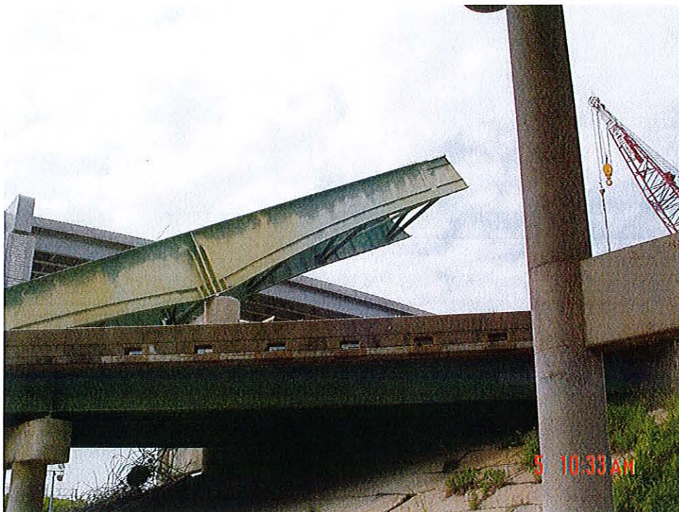
FIGURE 6 (Looking south, collapsed girder framing bent no. 3)
