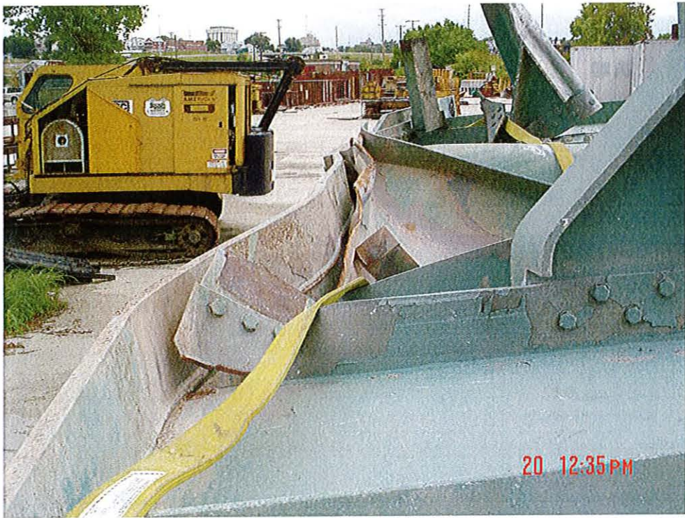
FIGURE 25 (Twisted top flange of the girder)
