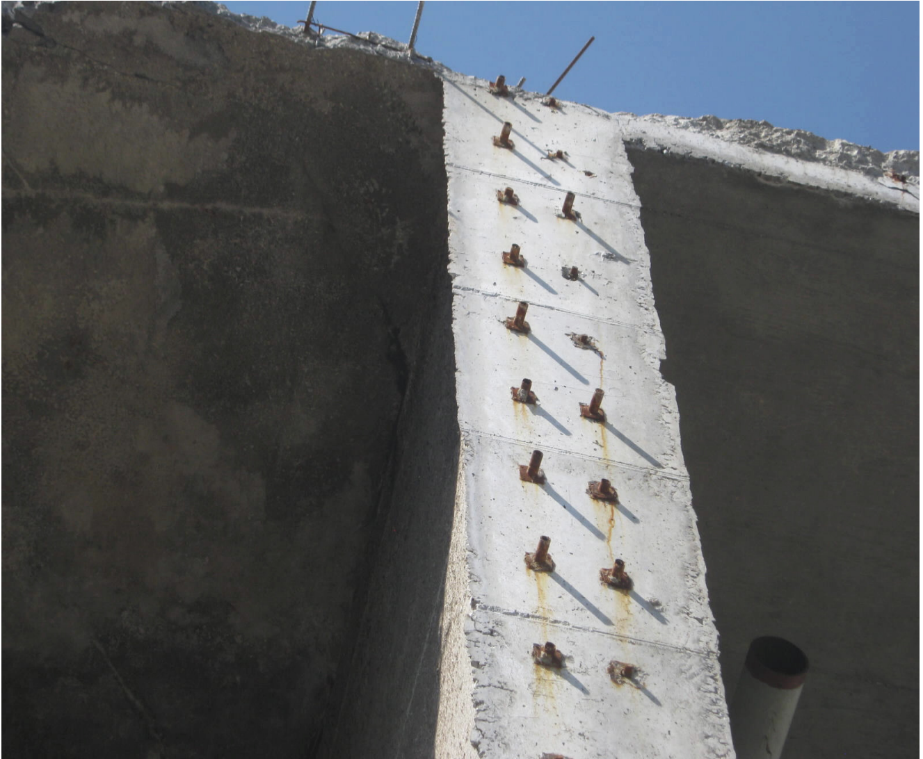
Fig. 3 Rebar Couplers used between the Baffle wall and the East Wall (Typical)
