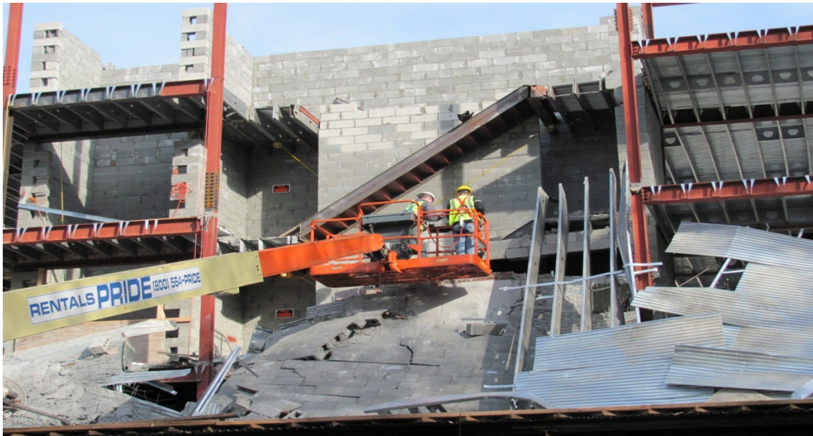
Fig. 6 Collapsed front face of the shear core wall.
