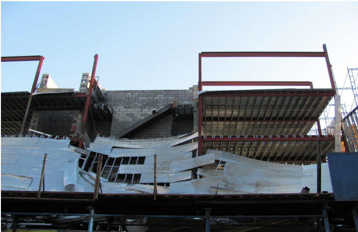
Fig. 5 Collapsed front bay of the building.
