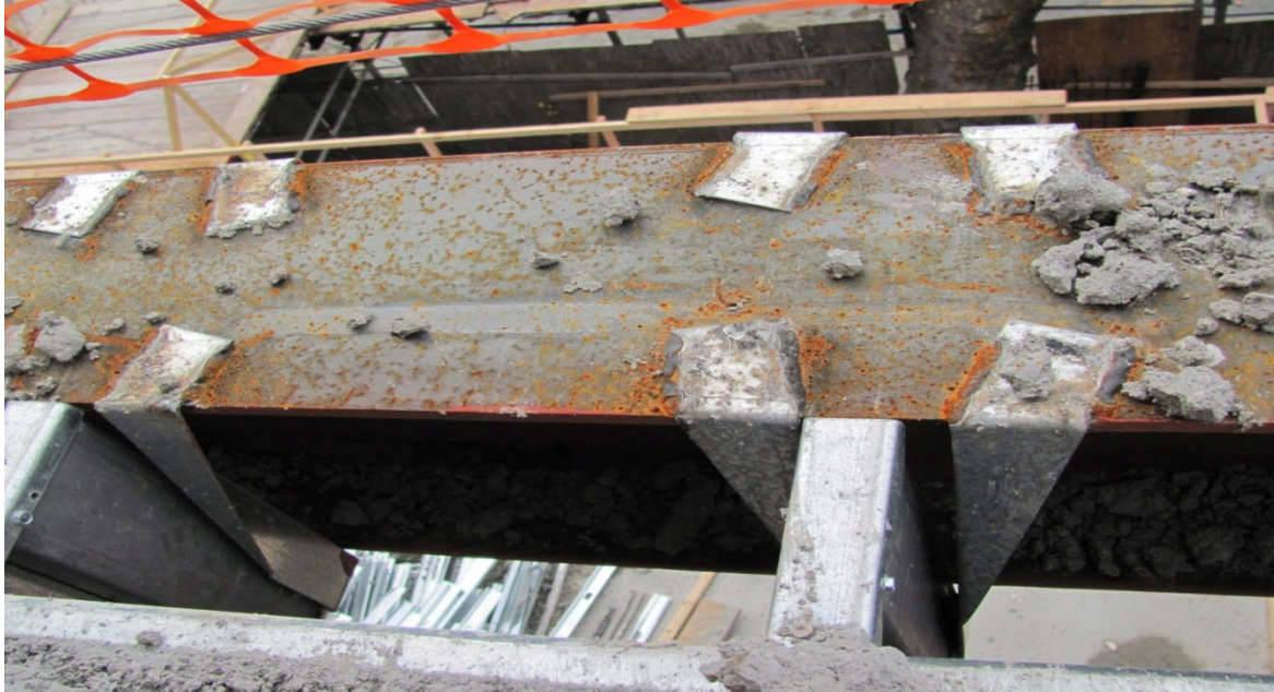
Fig. 4 Bridle hangers welded to a wide-flange steel beam and supporting floor C-joists.
