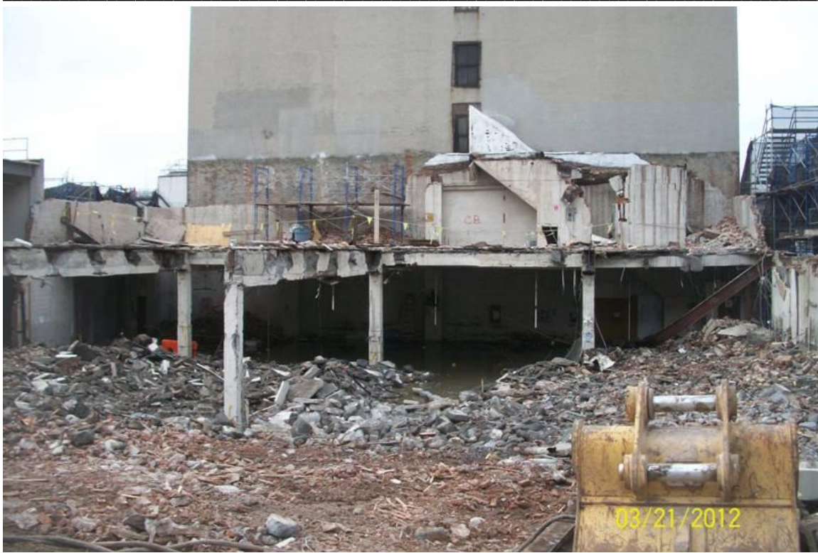
Figure 7 Second Floor Framing as it existed one day prior to the collapse
