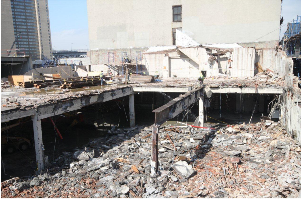
Figure 5 Second Floor Framing as it existed prior to the collapse
