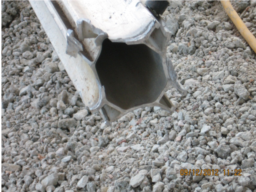
Figure 14. Another view of the failure condition of the welded connection at the end of a post shore.
