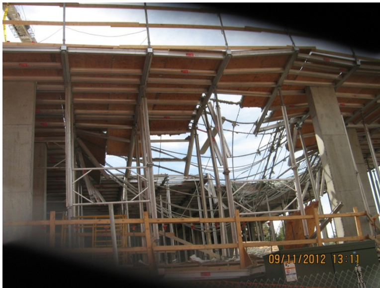
Figure 5. Collapsed shoring (Looking from the ground level toward the south).
