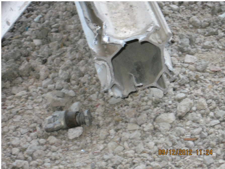
Figure 13. Failure condition of the welded connection at the end of a post shore.
