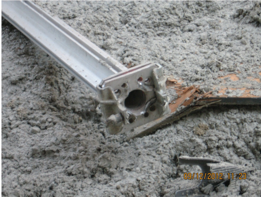
Figure 12. Condition of the splice plates after the failure of the post shore. Note that the two splice plates were located at the mid-height of the post shore.
