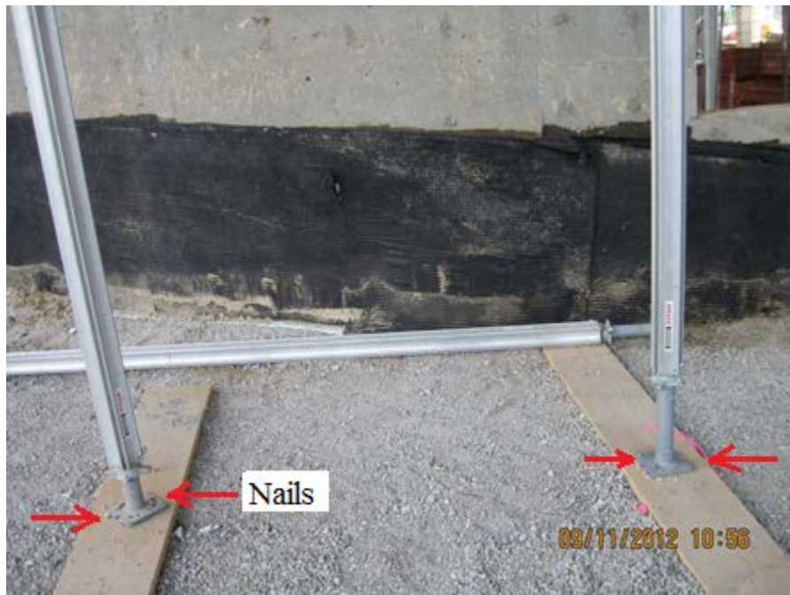
Figure 10. Base support condition of shores near the collapsed area.
