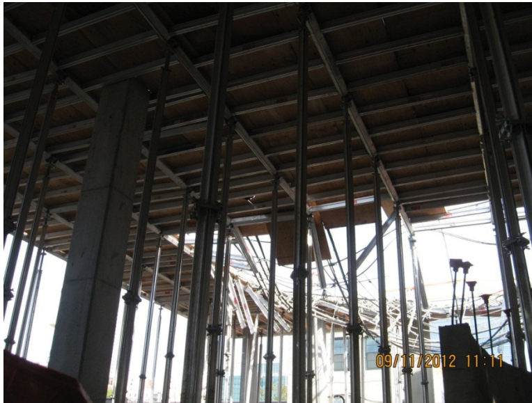
Figure 4. Collapsed shoring (Looking from the ground level toward the north).
