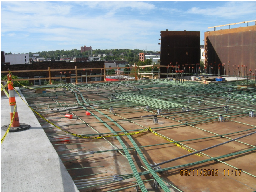
Figure 9. Concrete forming and reinforcement at the second level (Looking toward the south).
