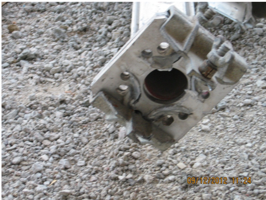
Figure 15. Failure condition of the welded connection at the splice plate. Note that this splice plate was located at the mid-height of the post shore.
