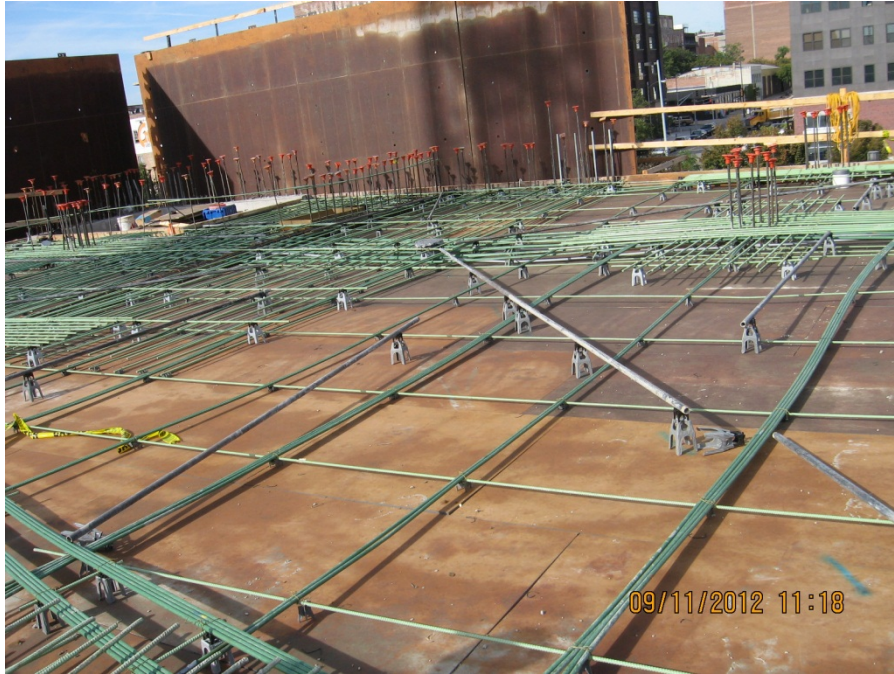
Figure 8. Concrete forming and reinforcement at the second level (Looking toward the southwest).
