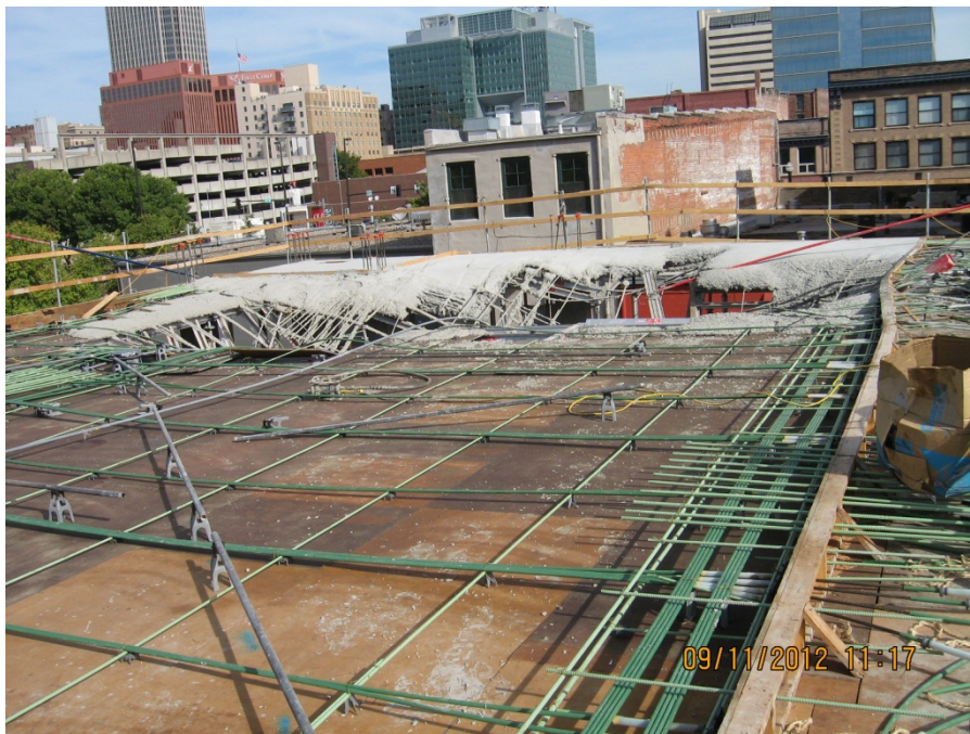
Figure 7. Collapsed concrete forming at the second level (Looking toward the north).
