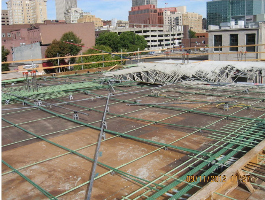
Figure 6. Collapsed concrete forming at the second level (Looking toward the northwest).
