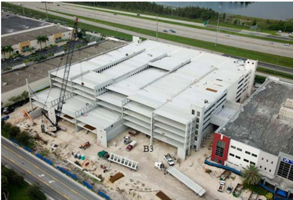
Fig. 20 – Pre-incident aerial photo (Progress as of 09/25/12)
