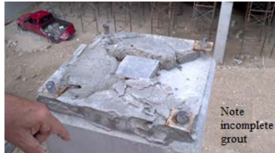
Fig. 57 – Close-up of the grout at splice of B4 column
