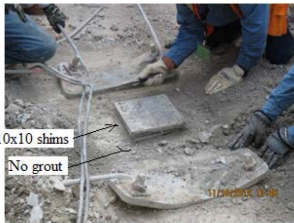
Fig. 47 – B3 column base plate and shims
