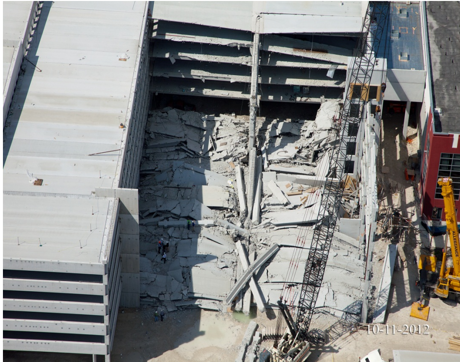
Fig. 15 – Aerial view of the collapse looking west
