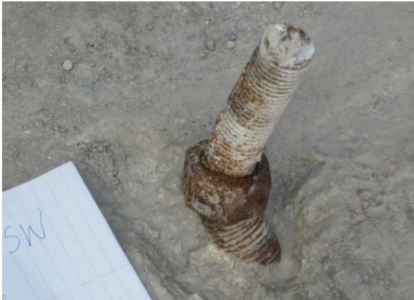
Fig. 50 – Deformed SW anchor bolt
