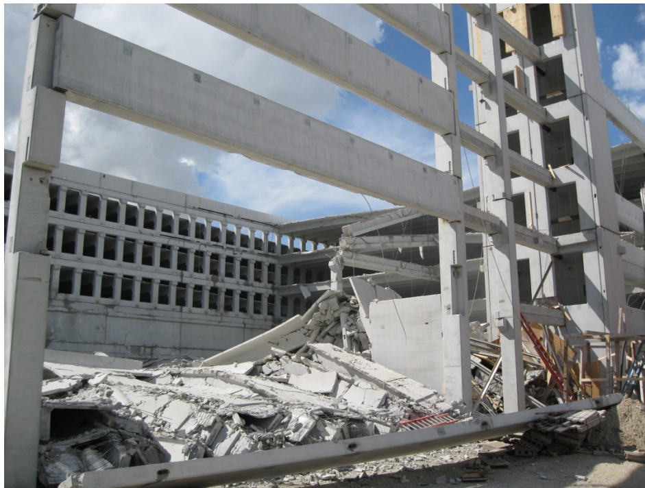
Fig. 14 – Another view of the collapse looking south
