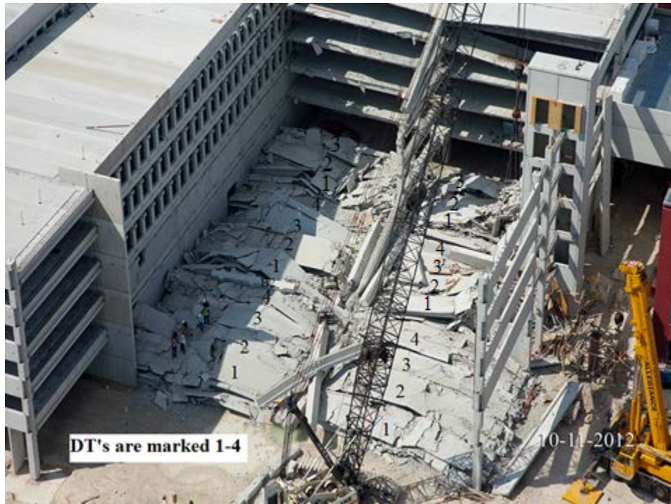
Fig. 19 – Some of the fallen DT's
