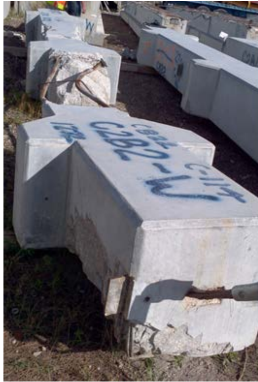
Fig. 33 – Column B2 shattered between level 6 and 5
