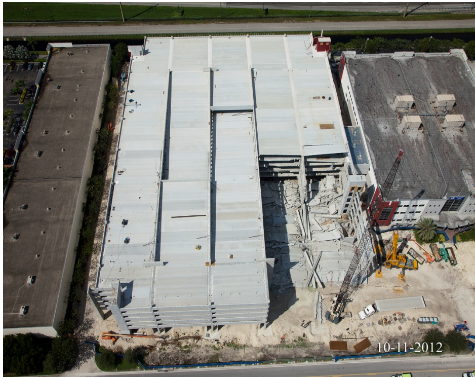
Fig. 11 – Aerial view of the collapse looking west
