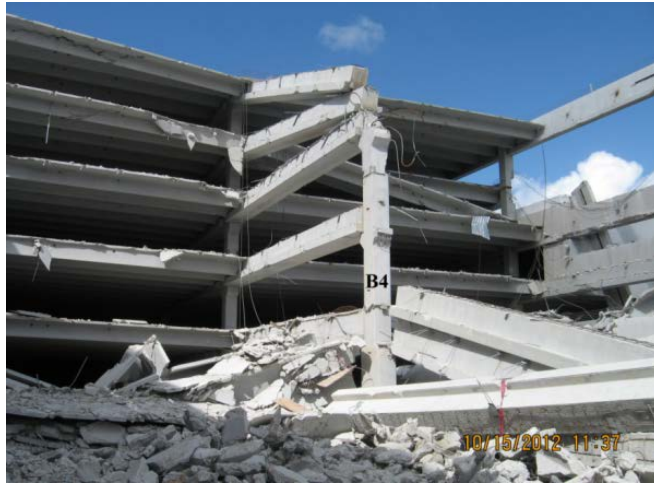
Fig. 52 – Column B4 remained standing after collapse
