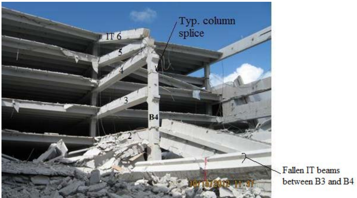
Fig. 17 – Column B4 after the collapse
