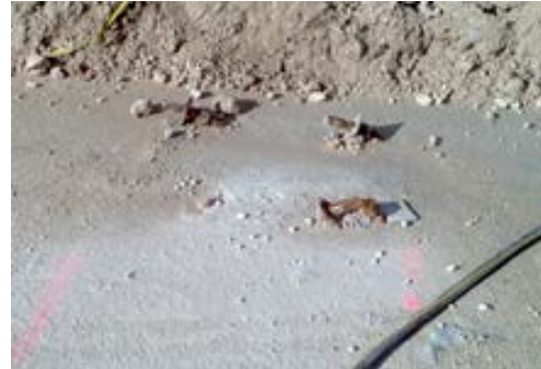
Fig. 62 – Base of column A3.3. No grout
