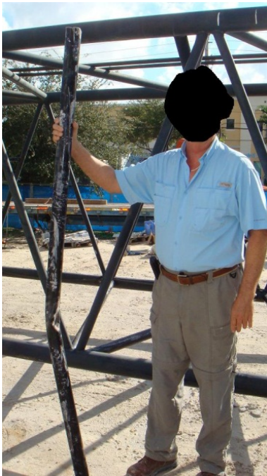
Fig. 30 – Damage to boom when crane hit B2 column (pre-collapse)
