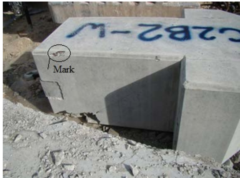
Fig. 31 – Column B2 marks after crane hit
