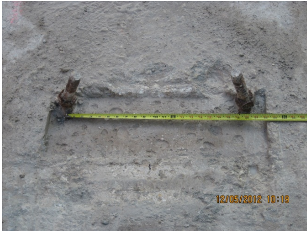
Fig. 48 – Bent anchor bolts
