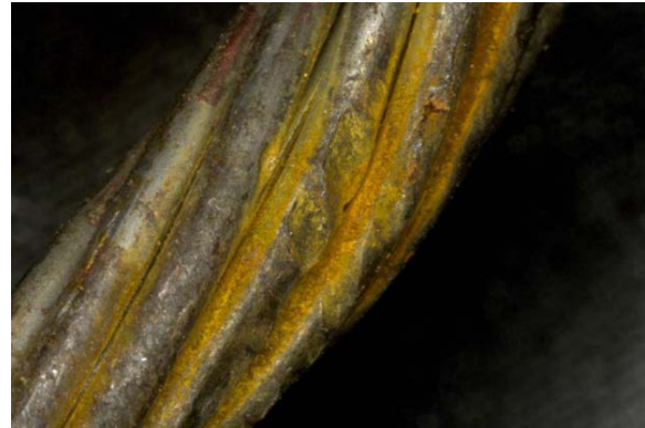
Figure 48: Rust/yellow substance on top of damaged wires
