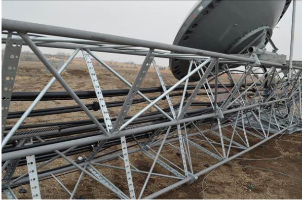
Figure 14 –New Tower after collapse
