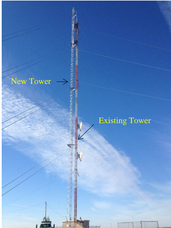
Figure 10 –New and existing tower
