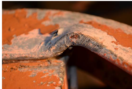
Figure 56 – Cuts and bruises from abrasion of wire rope
