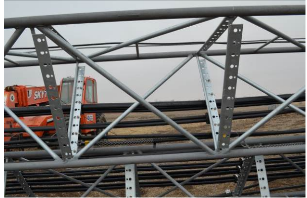
Figure 15 –New Tower after collapse
