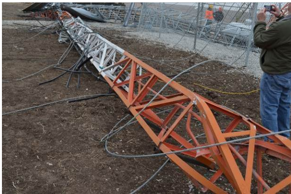
Figure 6 – Existing Tower on the field after collapse
