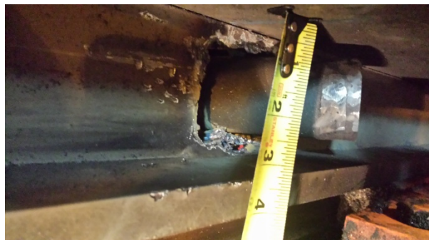
Fig 12 – Safety pin and the oversized hole
