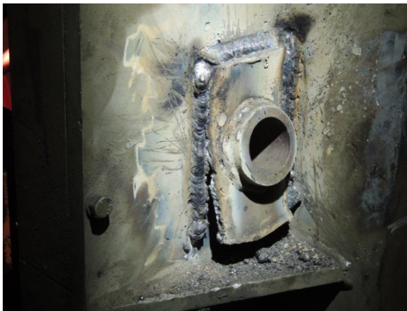
Fig. 9 - Failed weld and the bracket
