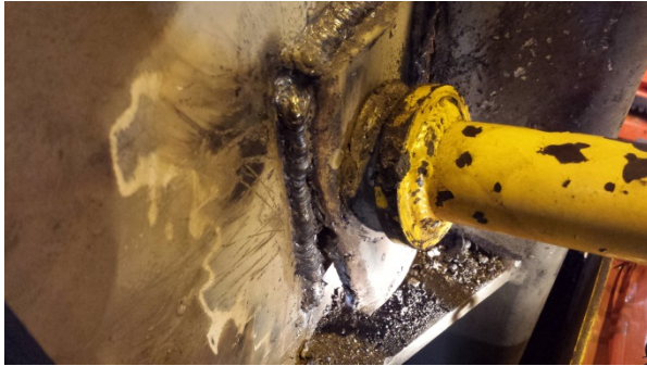
Fig. 7 - Failed weld, bracket and safety pin
