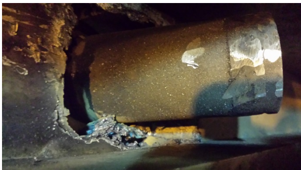
Fig. 11 - Safety pin and the oversized hole
