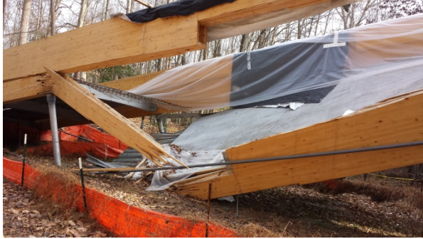
Fig. 40 – View of the collapsed girders
