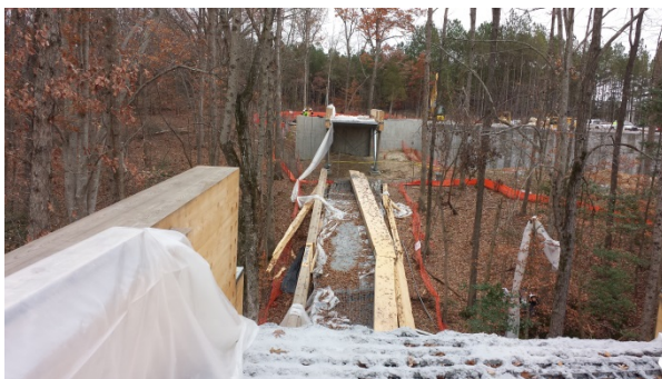
Fig. 23 – View of the collapsed girders
