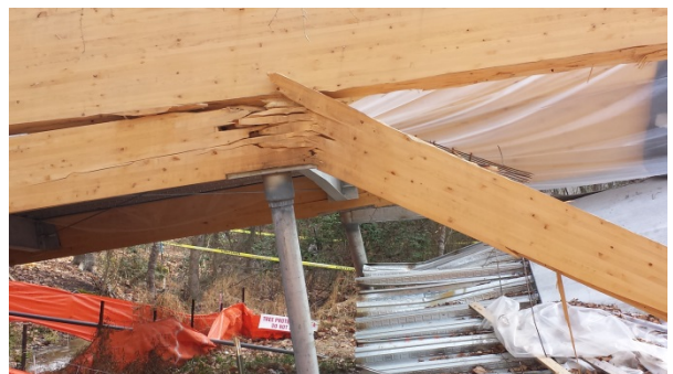
Fig. 39 – View of the collapsed girders
