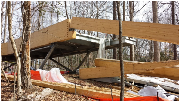
Fig. 34 – View of the collapsed girders
