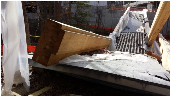
Fig. 42 – View of the collapsed girders
