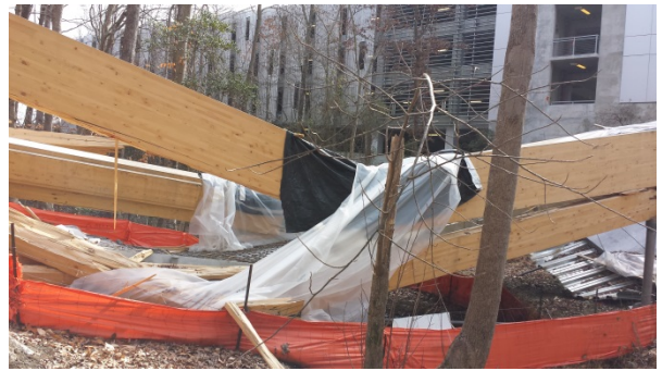
Fig. 35 – View of the collapsed girders
