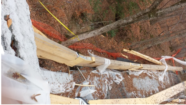
Fig. 25 – View of the collapsed girders
