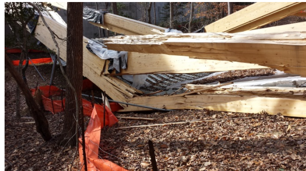
Fig. 43 – View of the collapsed girders
