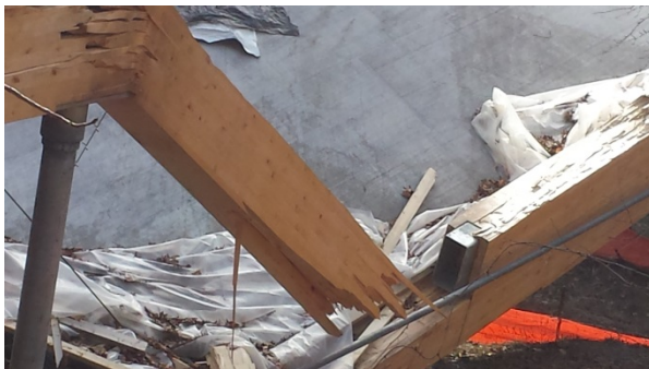
Fig. 36 – View of the collapsed girders
