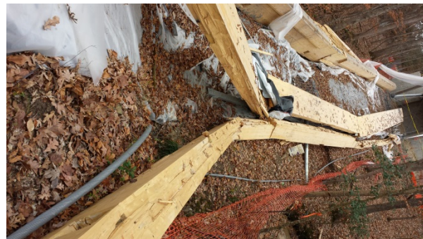
Fig. 28 – View of the collapsed girders
