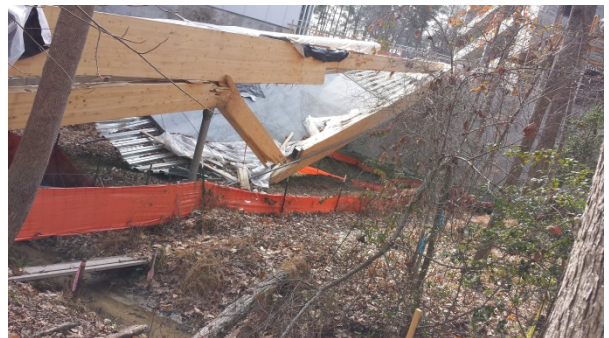
Fig. 37 – View of the collapsed girders
