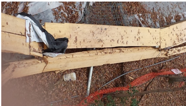
Fig. 27 – View of the collapsed girders
