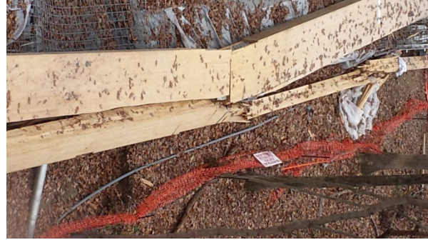
Fig. 26 – View of the collapsed girders
