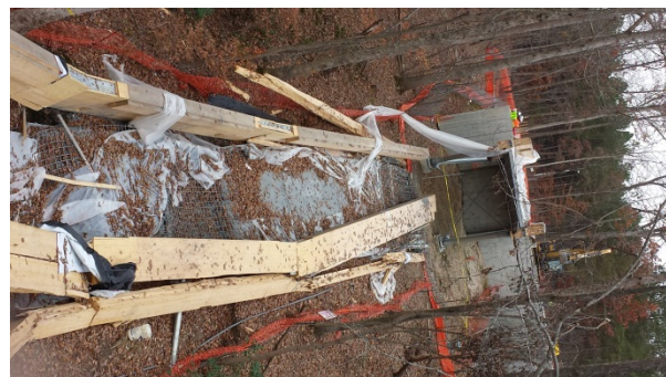
Fig. 24 – View of the collapsed girders
