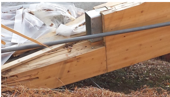
Fig. 38 – View of the collapsed girders
