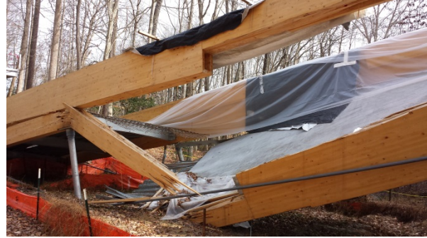
Fig. 41 – View of the collapsed girders
