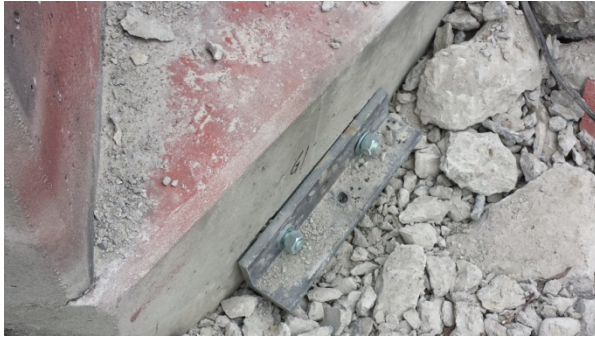
Figure 19 – 4x4x3/4" angle anchored to abutment #2 with Hilti anchors to prevent uplift of the girders
