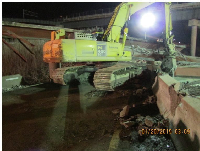
Figure 12 – Excavator after the collapse
