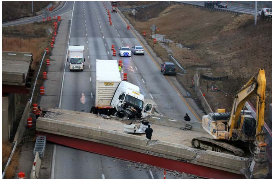
Figure 9 – Bridge center span with excavator collapsed onto I-75S (taken from the web)
