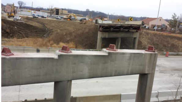
Figure 13 – Bridge piers after the incident
