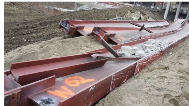
Figure 16 – Failed girders after collapse
