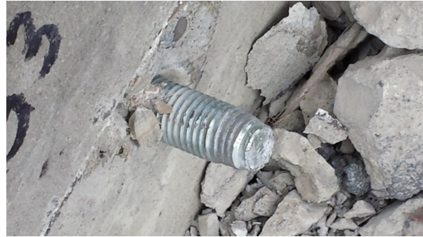
Figure 20 – Failed Hilti anchor
