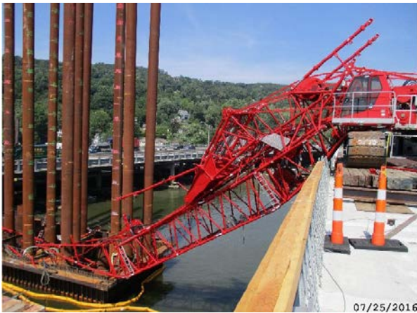
Taken from Thornton Tomasetti inspection report Fig. 22 – Shows the collapsed crane
