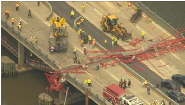
Taken from WestchesterNews Fig. 18 – Shows crane collapsed onto the existing bridge
