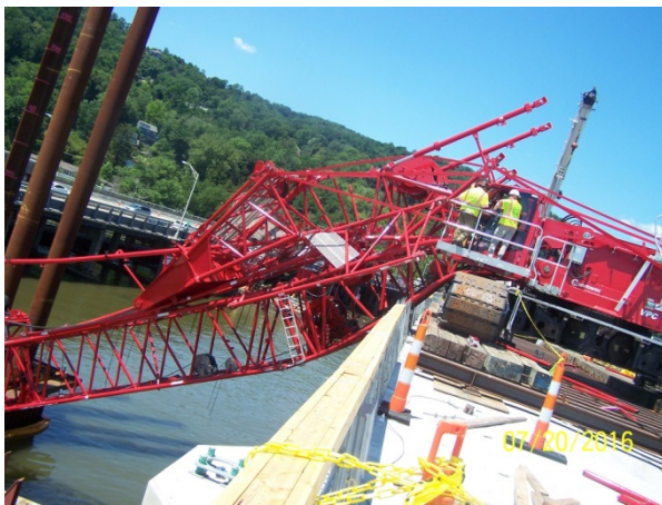
Fig. 20 – Shows the collapsed crane
