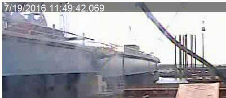
(shows that the Hammer was not attached to the pile at 11:49:42 a.m.)
