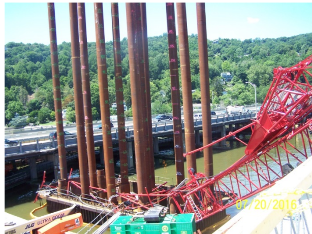
Fig. 19 - Shows the collapsed crane, piles and cofferdam
