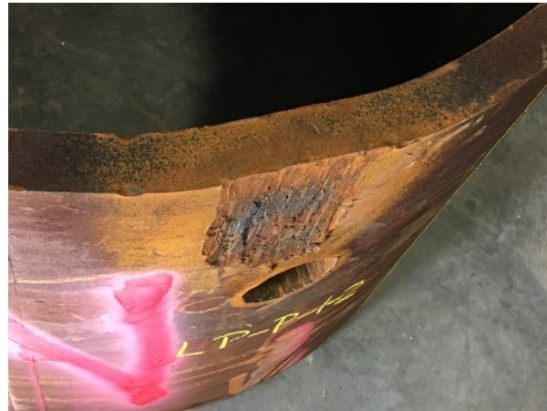
Fig. 35 – Mark on the north side of pile #1
