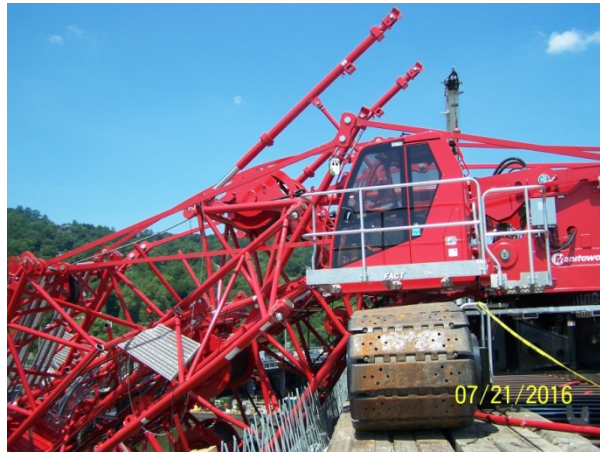
Fig. 23 – Shows the collapsed crane
