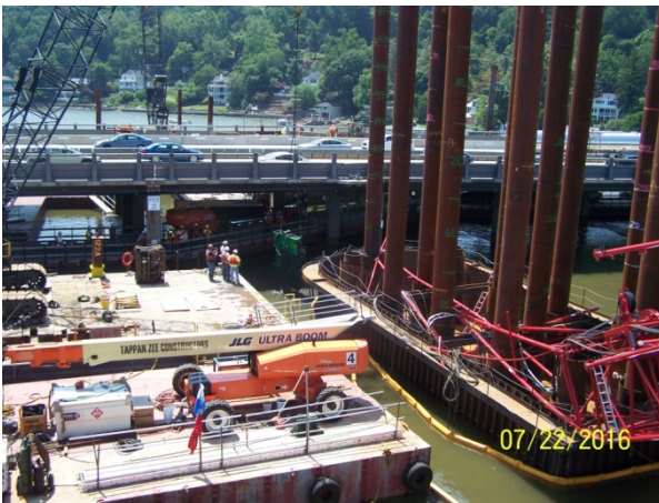
Fig. 24 – Collapsed crane, piles and cofferdam
