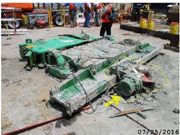
Taken from Thornton Tomasetti inspection report Fig. 27 - Vibratory Hammer recovered from water (Note: one clamp is missing)
