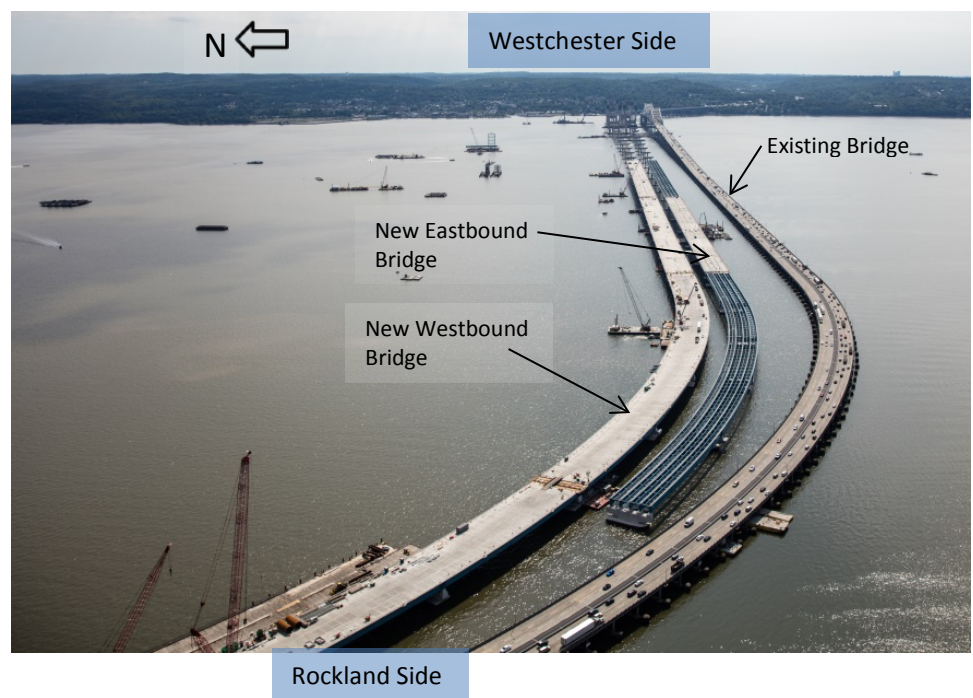
Taken from the New NY Bridge website http://www.newnybridge.com/photo/ Fig. 5 – Project progress photo (June 24, 2016)
