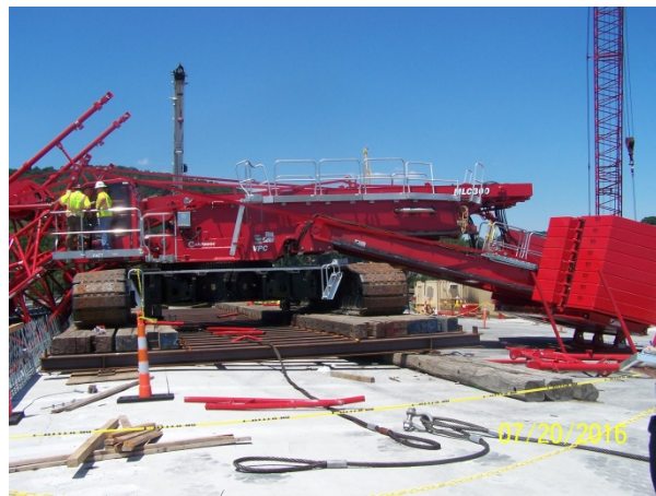
Fig. 21 – Shows the collapsed crane
