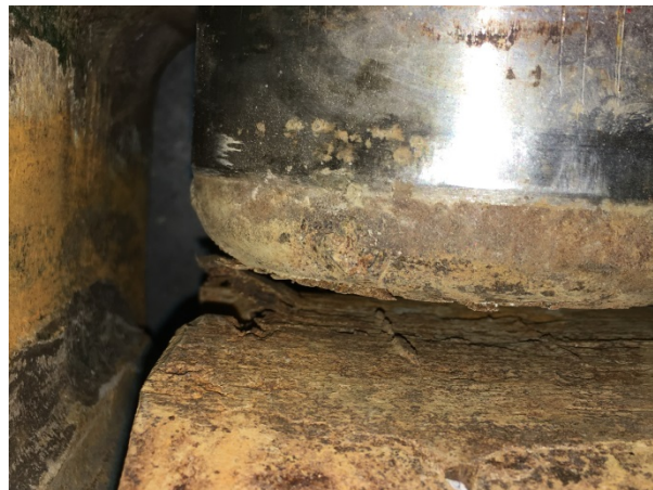
Fig. 41 – Close-up of corroded removable bearing plate
