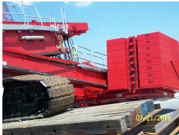
Fig. 25 – Collapsed crane with counterweight
