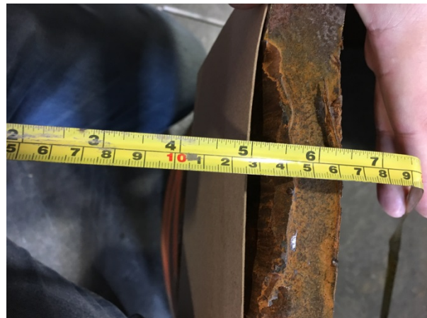
Fig. 37 – Deep indentation on the south side of pile #1
