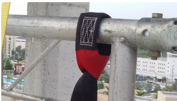
Fig. 31 – PFAS tied to the bracing of a table.
