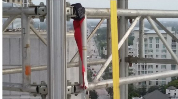
Fig. 30 – PFAS tied to the bracing of a table.
