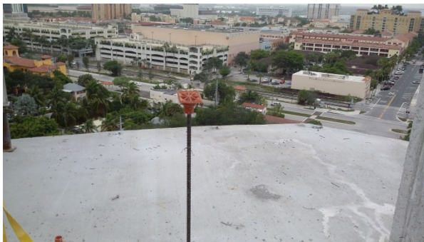
Fig. 16 – Screw pulled out from concrete.
