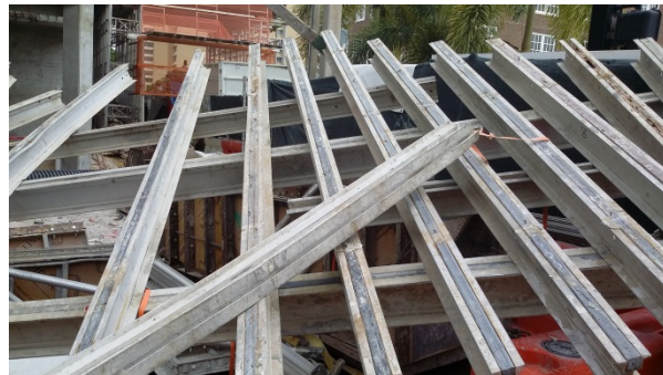
Fig. 14 – Collapse photo. (T27 after collapse)
