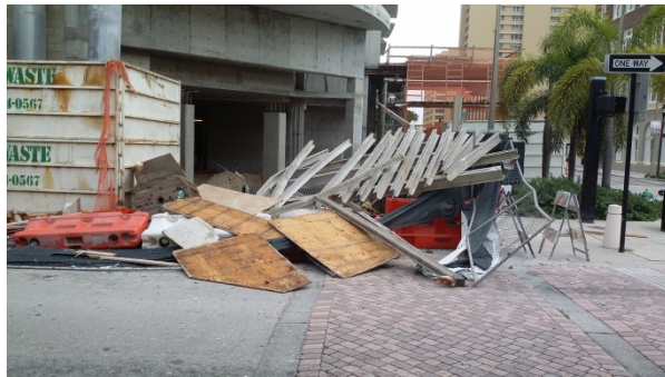
Fig. 13 – Collapse photo. (T27 after collapse)
