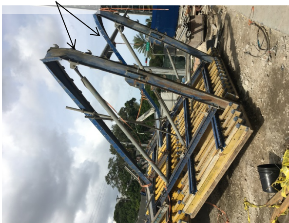
Fig. 15 – One of the failed platforms
