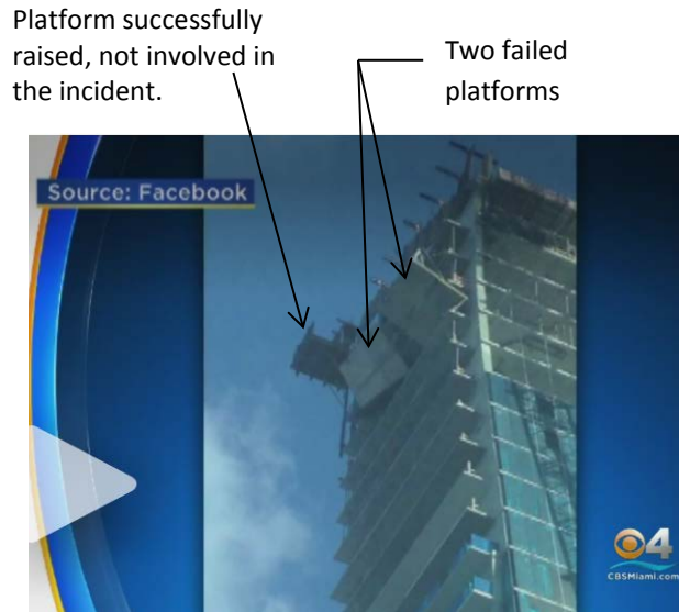
Taken from CBS Miami Fig. 9 – Failed platforms
