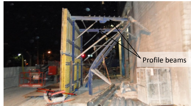
Fig. 16 – Other failed platform
