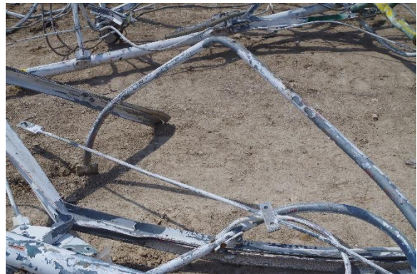
Figure 9. Bent Redundant Member at 105' Tower Elevation
