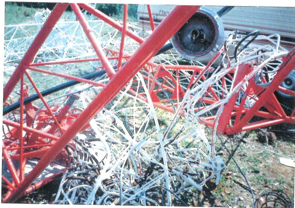
The collapsed tower structure Figure 1.4
