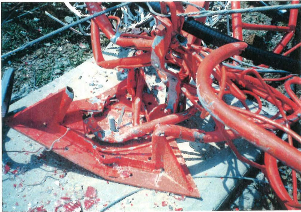
The Buckled Middle Tower (Section 16)-top photo The Rotated/Bent Tower Base Plate- bottom photo
