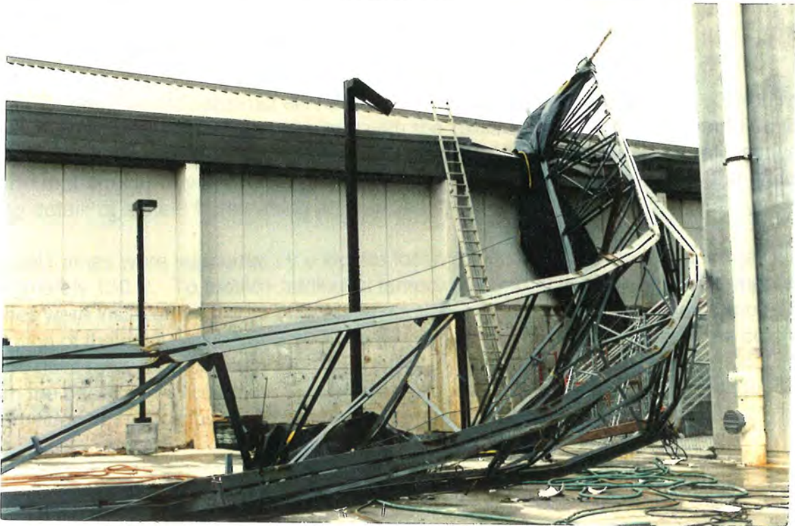
South End of Collapsed Joists Resting On Roof of Student Gymnasium (Looking southeast) Figure 1.4
