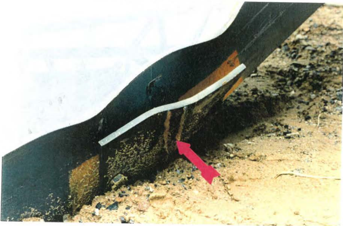
T1 Joist Bearing. Arrow shows location of failed weld on bearing plate.
