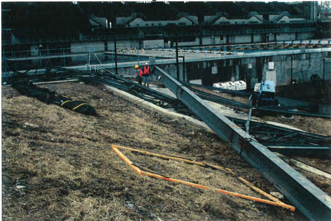
Frame and Paired Joists on Ground (Looking south-southwest; Existing pool in background) Figure 1.2
