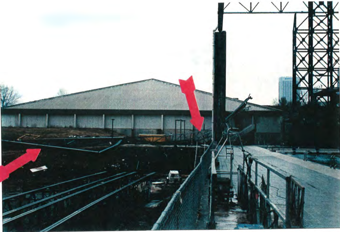
Failed Steel Joists and Frame (Arrows) (Looking east; Existing pool on right, Student Gymnasium in background) Figure 1.1
