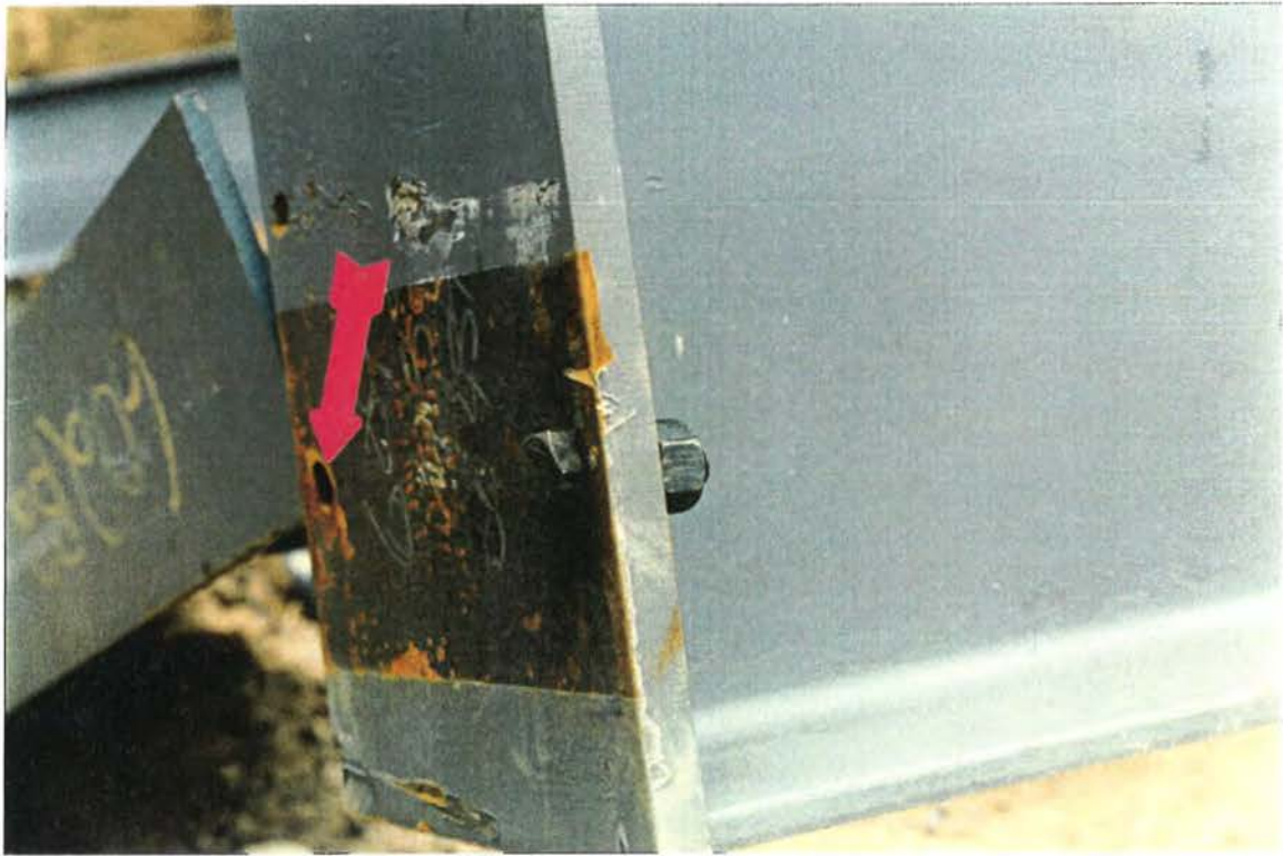
T2 Joist Bearing. Arrow indicates location of the failed bolt.
