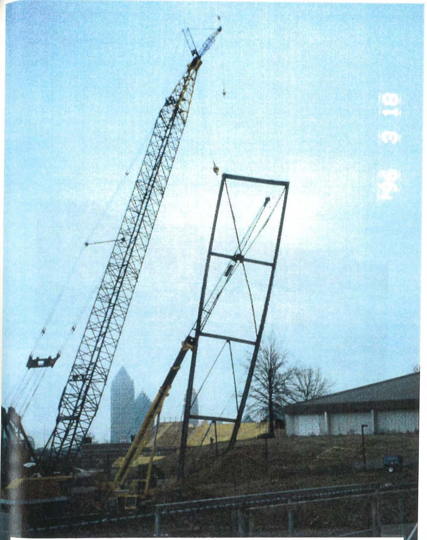
Figure 5.5 - Post Event Disposition of Frame With Crane Hoistline Attached
