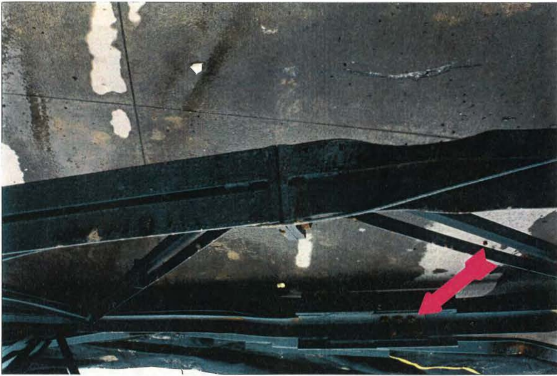
Top & Bottom Chord Center Splices (Looking West - Arrow Shows Bottom Chord Splice)
