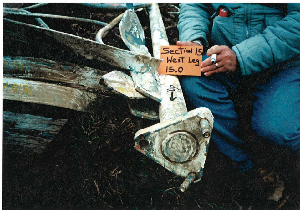
Gusset plate of diagonal 14.5a1 at the West leg. Connecting bolt missing, member intact.
