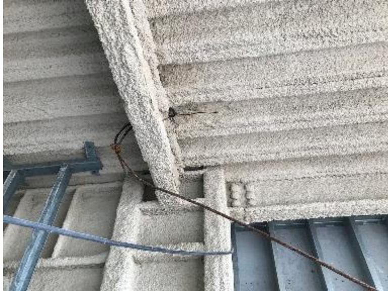
Figure 12: Broken wire rope where it went over a beam. There was no protection for the wire guy rope.
