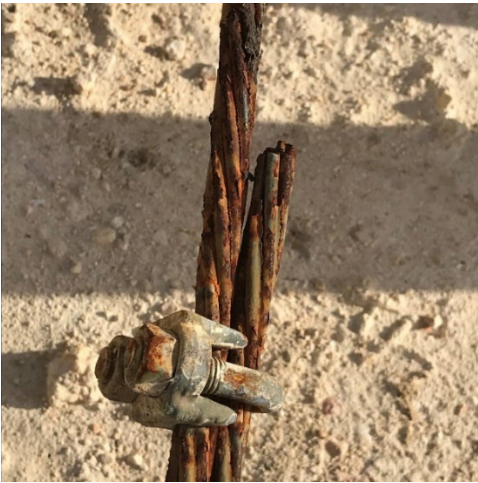
Figure 33 – Failed cable connections
