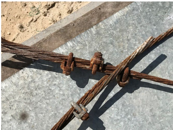
Figure 34 – Failed cable connections
