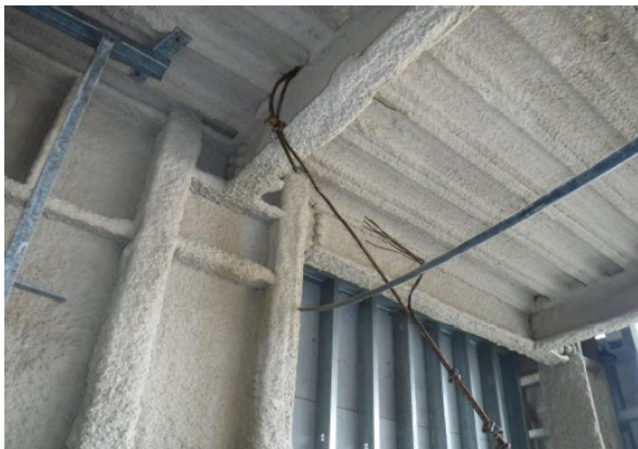
Figure 30 – Failed cable connections
