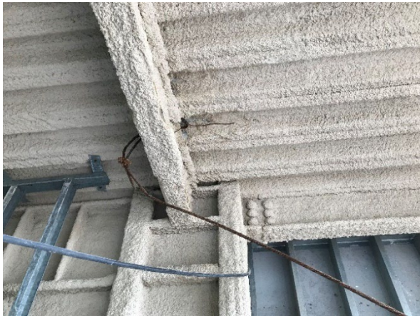
Figure 32 – Failed cable connections
