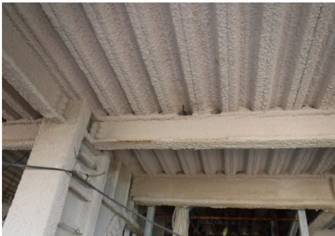
Figure 25 – Cables wrapped around hotel beam and column
