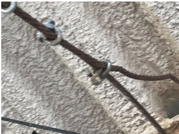
Figure 35 – Cable with kink that was used to support a scaffold on the fifth floor
