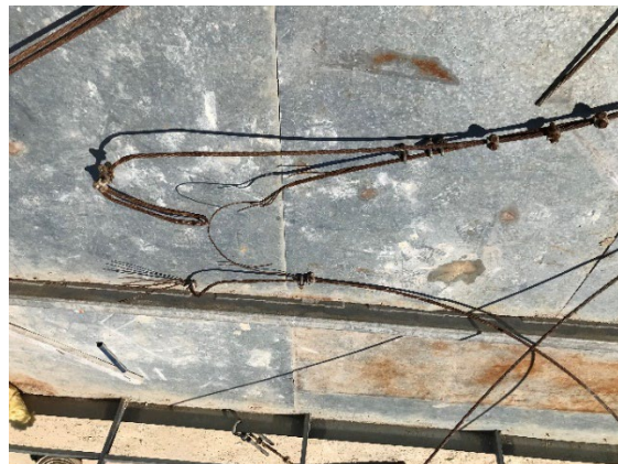
Figure 31 – Failed cable connections
