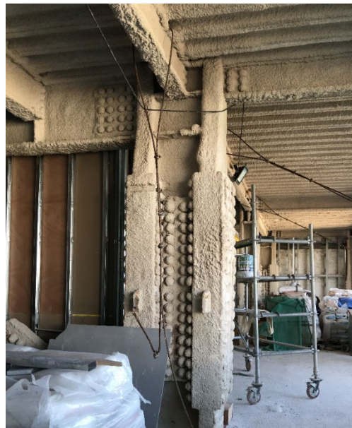
Figure 26 – Cable wrapped around hotel beam and column
