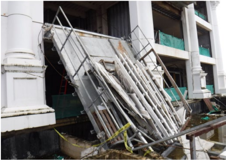
Figure 2 – Failed scaffold with material
