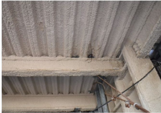
Figure 24 – Cable wrapped around hotel beam and column
