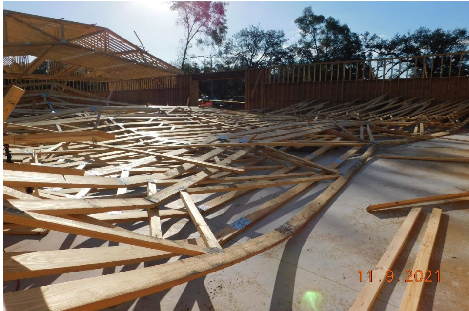
Figure 11 – Collapsed roof trusses – looking southeast
