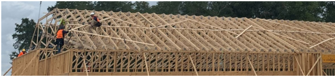
Figure 12 – Truss braces at the south side – looking north (Photo by WW Build)
