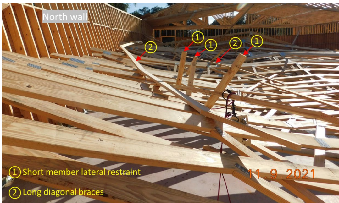
Figure 13 – Truss top chord braces at the north side after collapse – looking east
