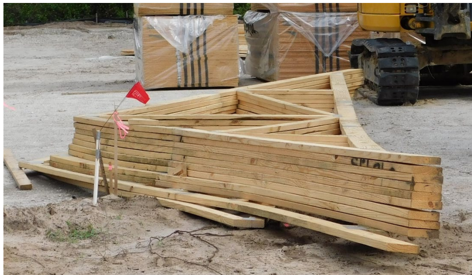
Figure 18 – Incorrect jobsite storage of trusses
