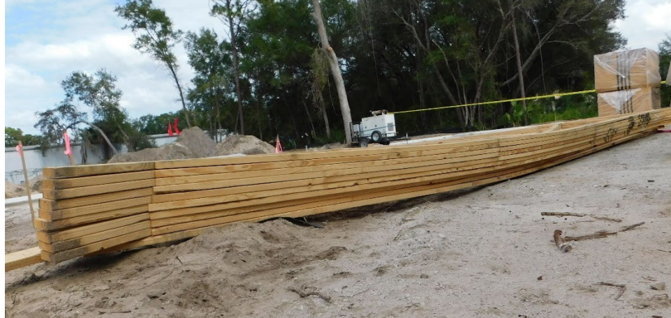
Figure 19 – Incorrect jobsite storage of trusses
