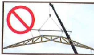
PHOTO B1-7 Spreader Bar is too short for this Truss.
