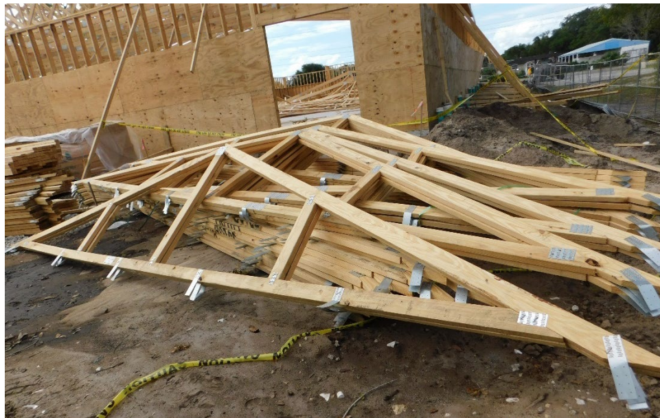
Figure 20 – Incorrect jobsite storage of trusses
