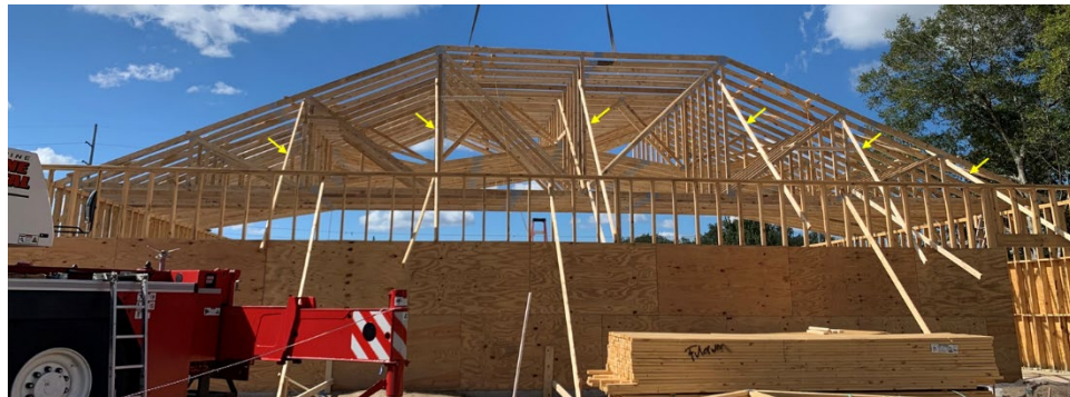
Figure 8 – Truss diagonal end braces at the east side – looking west (Photo by WW Build)
