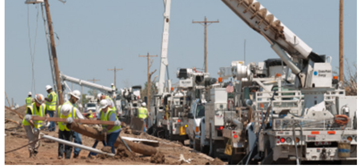
OG&E employees and mutual assistance crews work to repair damage from the May 2013 storms.
