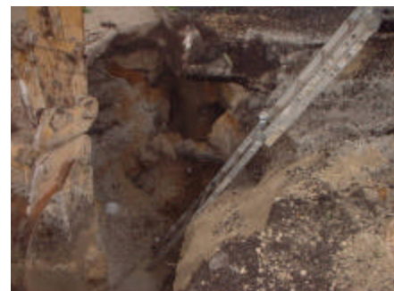
This is not a trench you would want to be in—even with a ladder.
