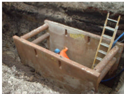
A trench box is being used—but what is wrong with this picture? Hint—what would happen if the soil on top collapsed?
