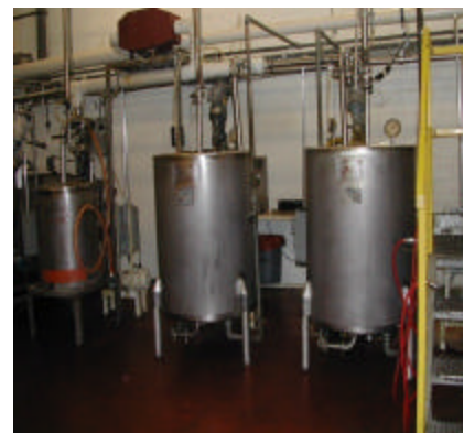
Flavor tank ventilation
